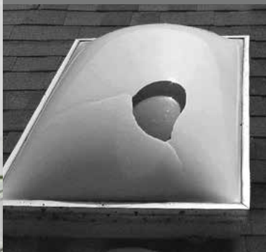
Old acrylic domes can be easily damaged.
